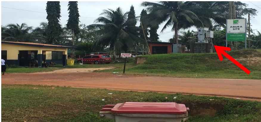
Plate 2. 1: Existing Transformer (arrowed) at the Abura Site
